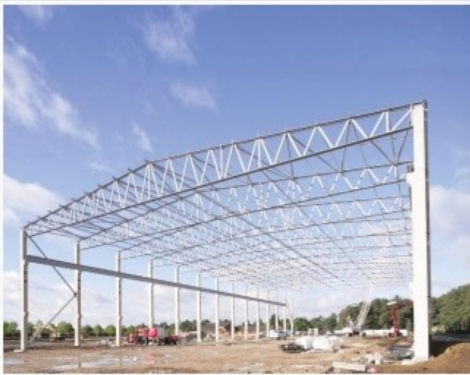
Bolted angles to form lightweight, long-span trusses
